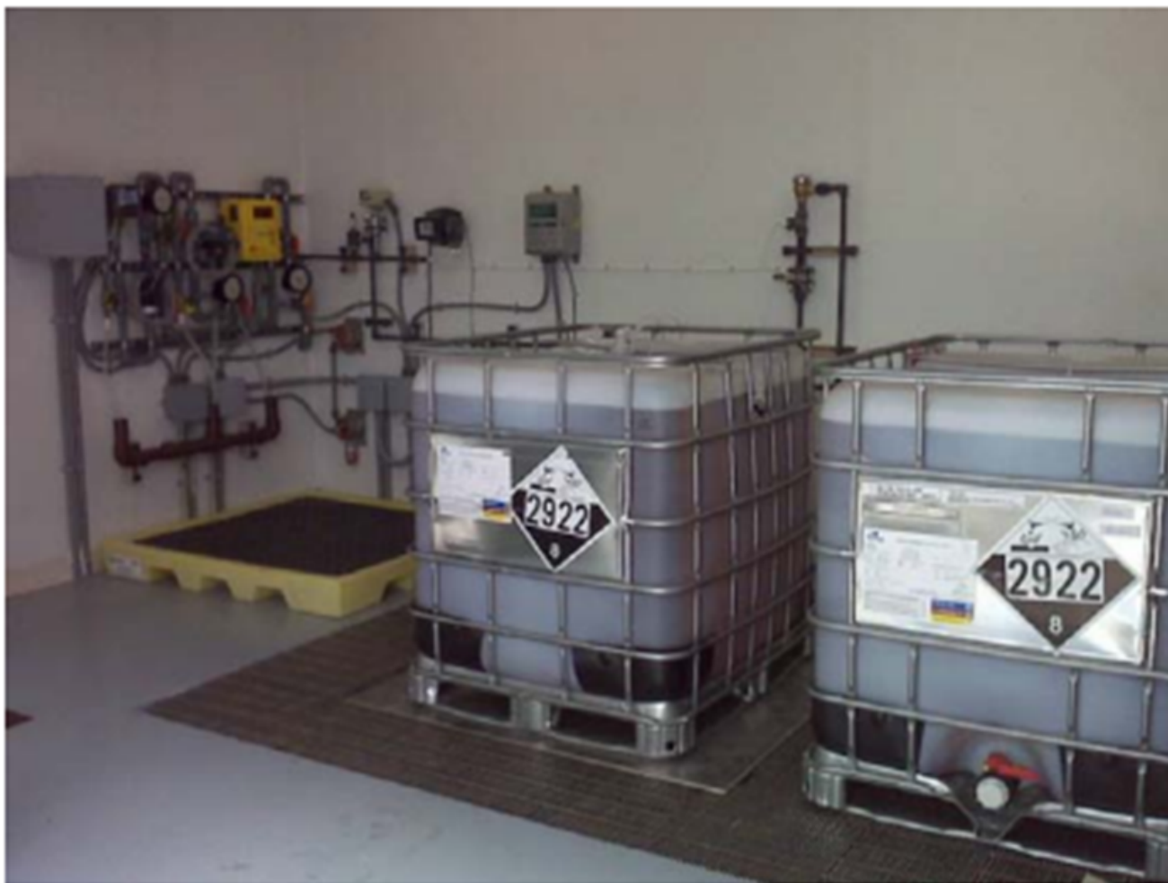
Figure 1. Photograph of the entire NaSH pretreatment system including the NaSH totes.
